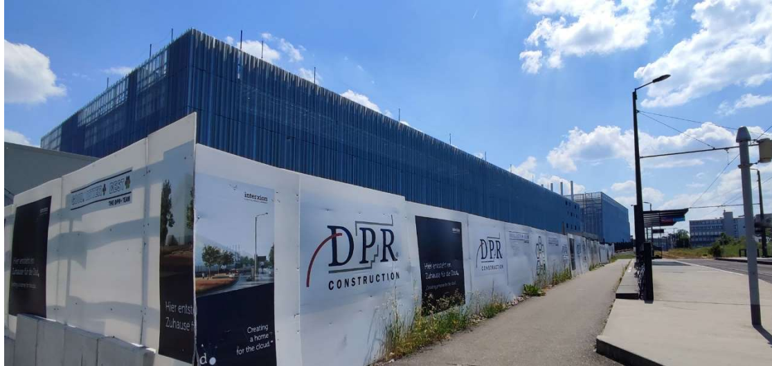
Figure 42. A “home for the cloud”. Perhaps, but also the enormous Interxion data centre buildings in the outskirts of Zürich. The tram station on the right looks minuscule in this photo.
